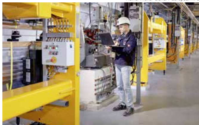
An engineer runs tests at the first fully installed undulator system in the European XFEL
