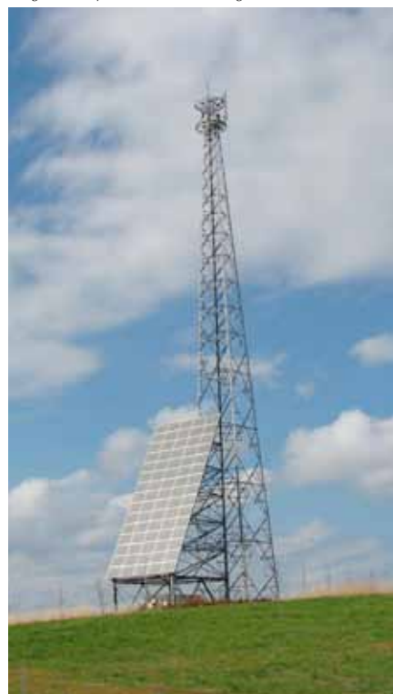
Mobile-phone base station powered by photovoltaics
