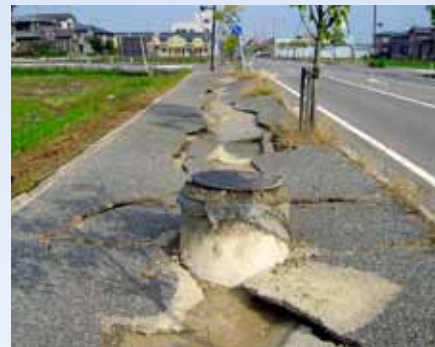
Earthquake damage to a pavement
