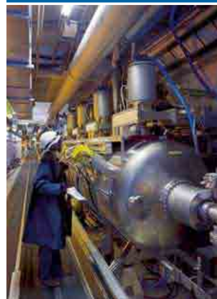
LHC superconducting accelerator cavity in the LHC tunnel
