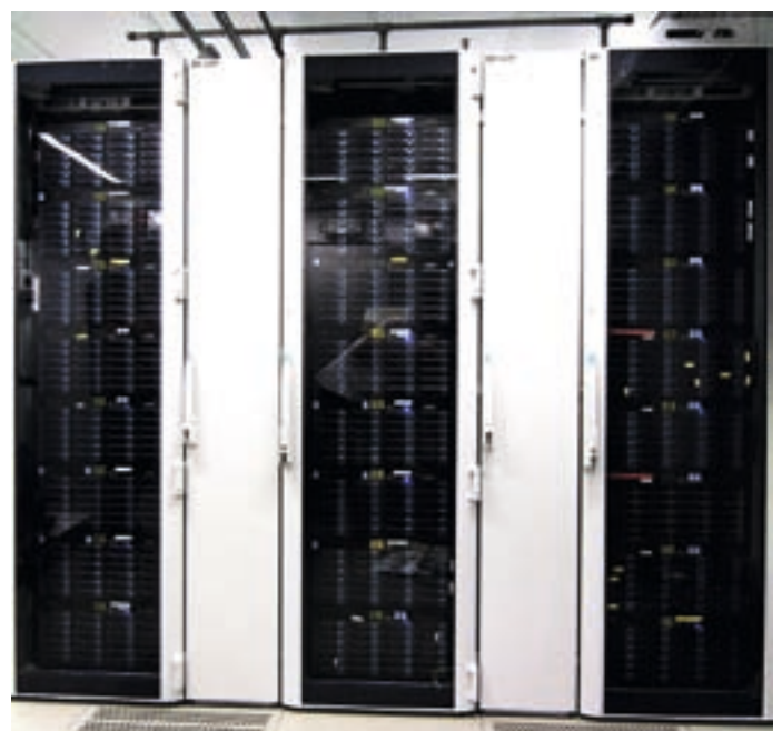
Figure 2: The current 24-machine NGAS cluster in its new location, the ESO data centre. Each of the three racks weighs about 1 000 kg and uses a sophisticated dual cooling system, located behind the narrow grey doors. The cluster can host up to 576 SATA disks. With the currently used 400 GB disks this translates to a total capacity of 156 TB in 48 RAID5 disk arrays.
