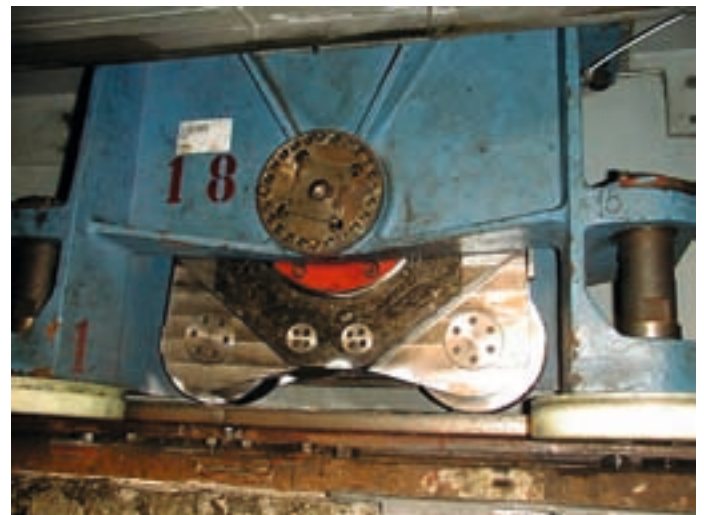
Figure 7: One of the eight new wheel units is shown in position attached to the dome.
