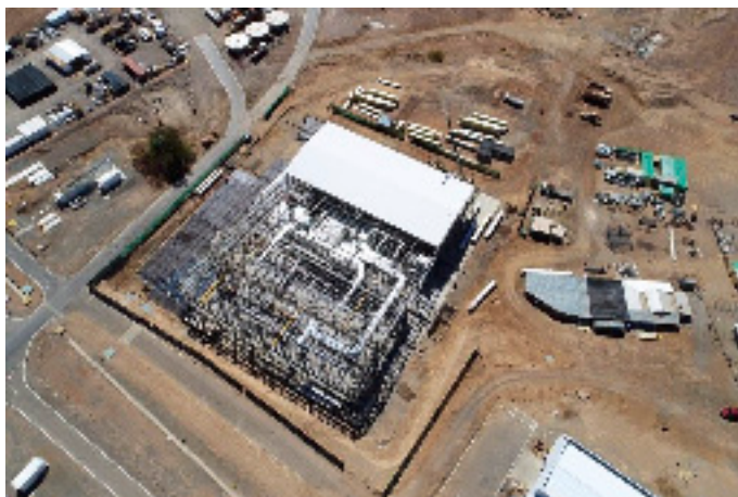
Left: Construction of the ELT Technical Facility (ETF) is progressing at Paranal with completion expected in 2020.
