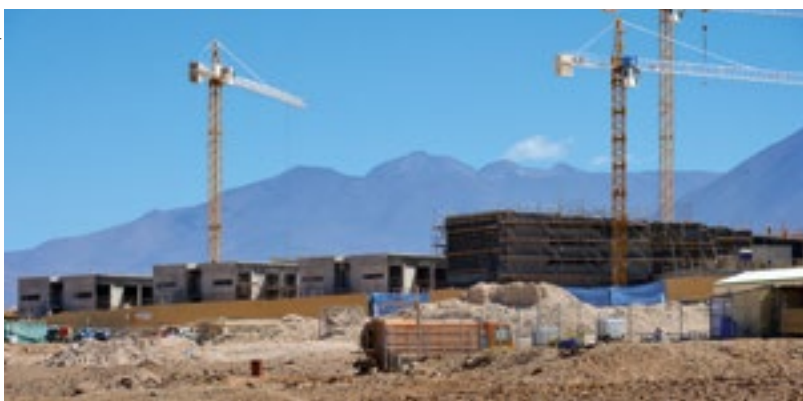
Construction of the ALMA Residencia started in February 2015 and was in an advanced state by the end of 2015.
