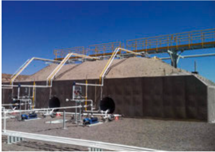
The LPG storage facility: the tanks are covered in sand for enhanced safety.
