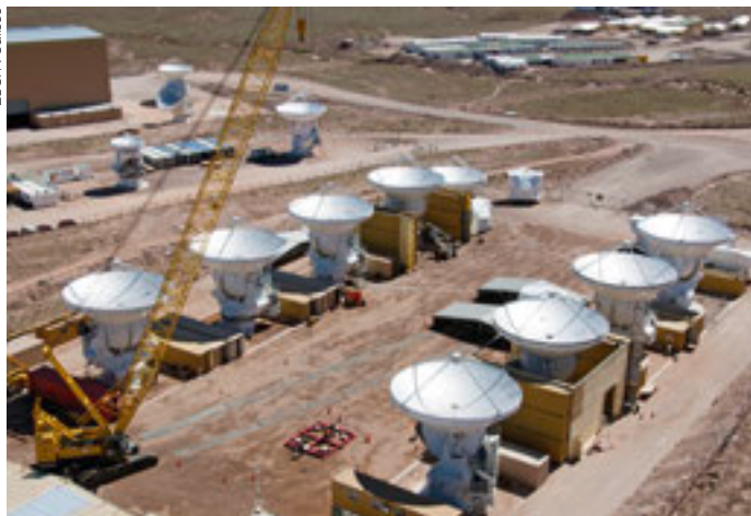
View of the AEM assembly area at OSF from the holography tower, with eight antennas in completion and four steel structures parked (August 2012).
