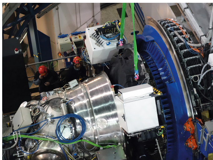
Installation of GRAAL on UT4. HAWK-I is the shiny metallic structure on the left while the blue part on the right is the Nasmyth A adapter/rotator. GRAAL is the black structure lying in between.
