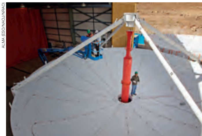
The first two back-up structures of the European ALMA antennas at the OSF.
